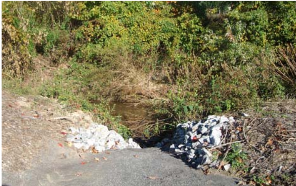
Storm Outlet to a Creek
